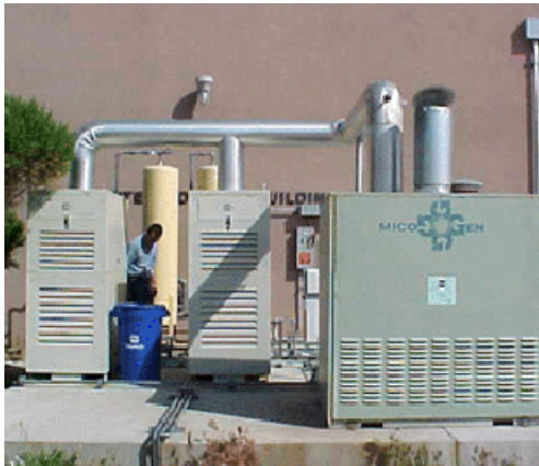
Figure 2.30: The Cogeneration System with two 30 kW Capstone MGTs (from ref. [55]).
